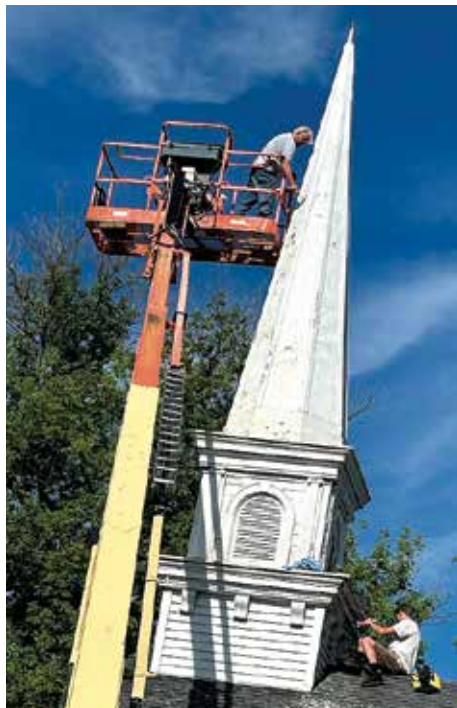
Photo courtesy of Don Sherman Over last weekend the steeple of Belleville Presbyterian Church was renovated. Church member Eric Gow and his assistant Gabriel Hardy worked on the steeple 62 feet in the air with the help of a cherry picker. A 24" tall cross made by welder Randy Dunkelberger was put on top.
