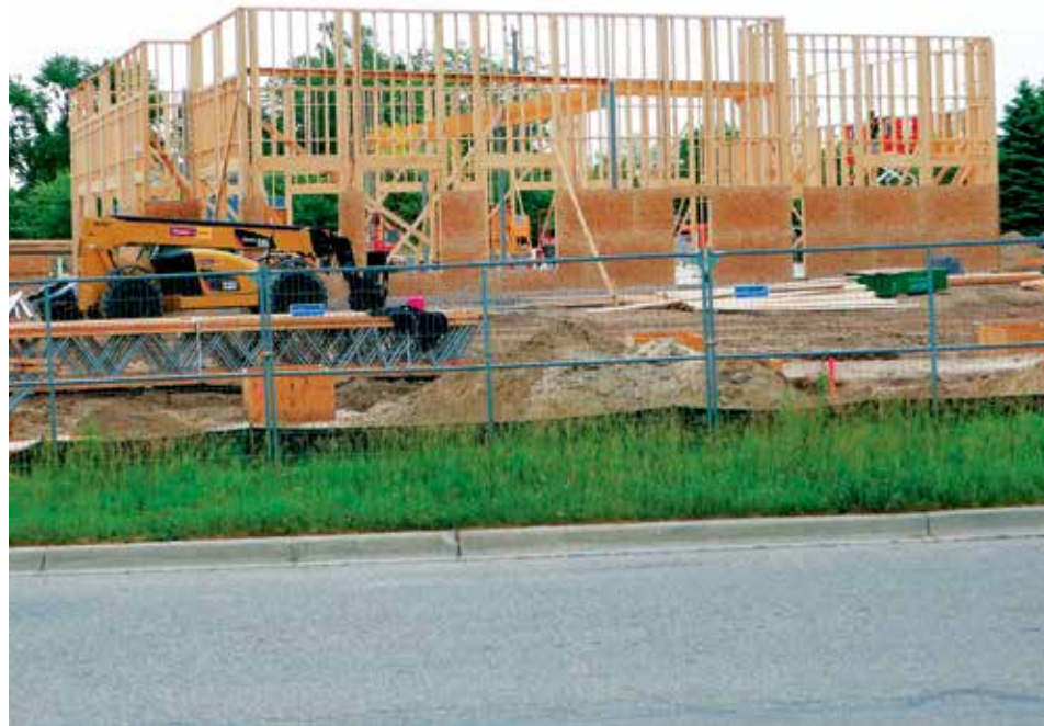
Independent photo by James Otzman Work continues on the new Chick-fil-A restaurant on Belleville Road. This photo was taken May 22.
