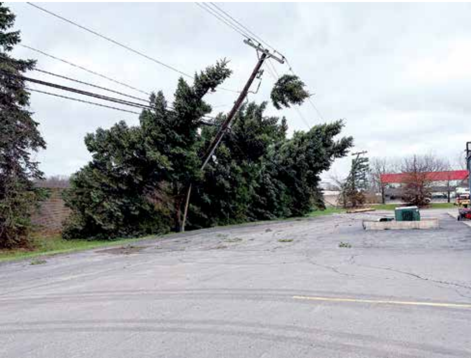
This photo from the National Weather Service shows storm damage behind JT's Pub and Grub on E. Huron River Dr. in Van Buren Township. LKQ Michigan's building is in the background.
