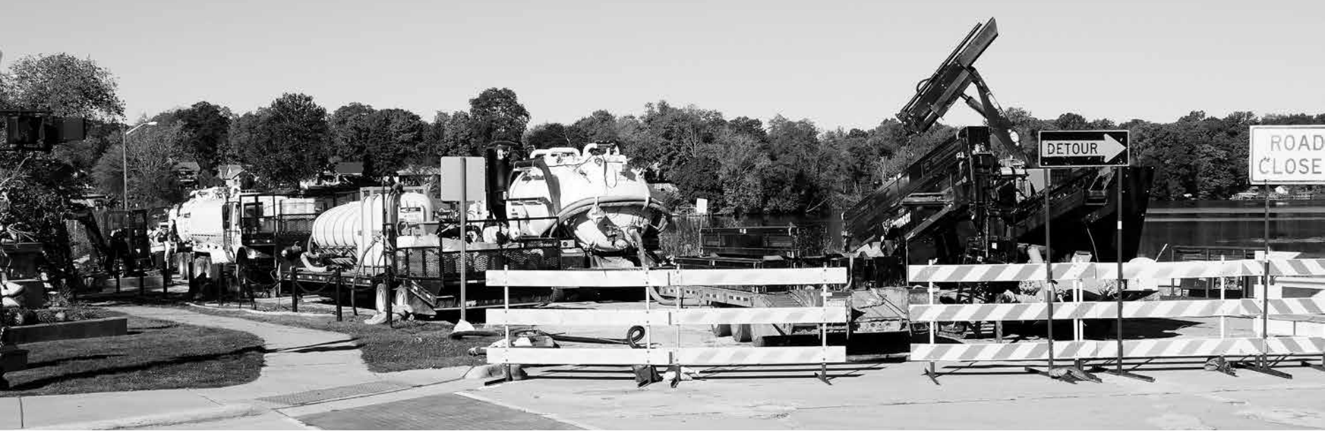
Independent photo by James Otzman DTE has gathered equipment at the Denton Road Bridge over Belleville Lake and will begin the underwater directional boring for its gas line. Van Buren Township Director of Municipal Services Ron Akers said DTE told him that it will take until the end of the year to complete its project. Then, the bridge is expected to be demolished in January.
